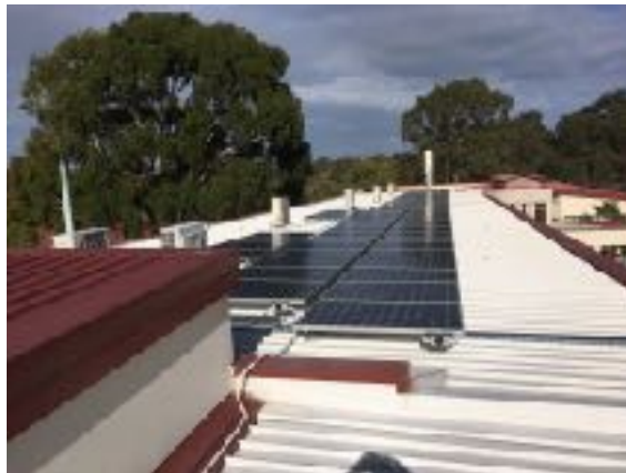
The new solar panels are in place and already
